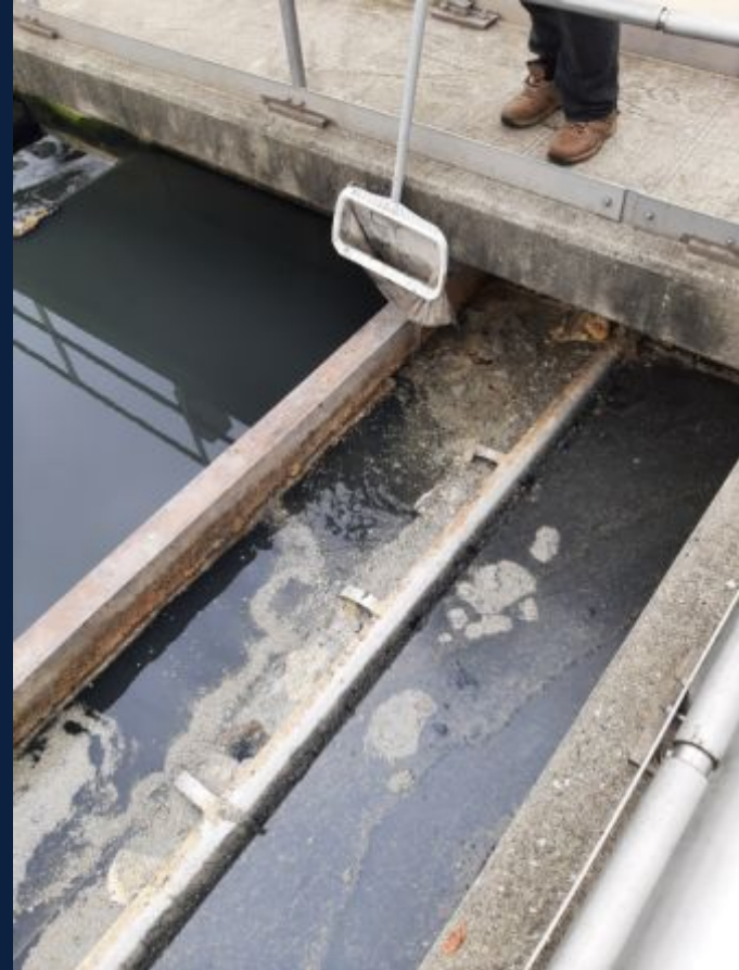
Manual FOG skimming at Primary Settling Tanks
